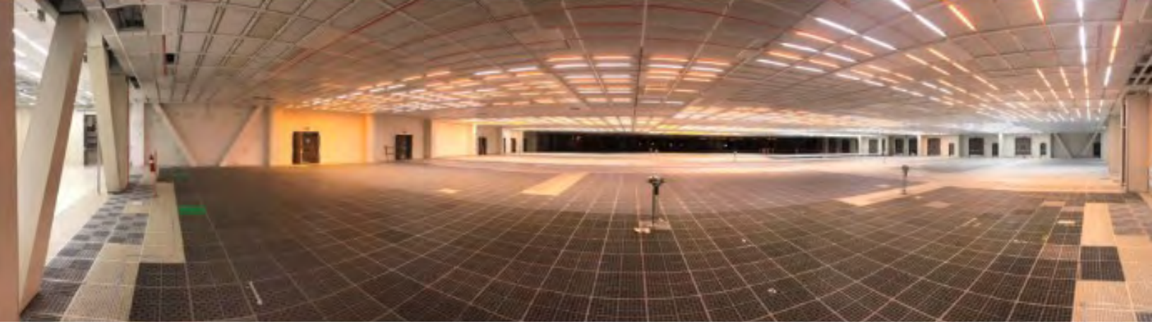
4' Raised Floor - 1615 High Tech Way
